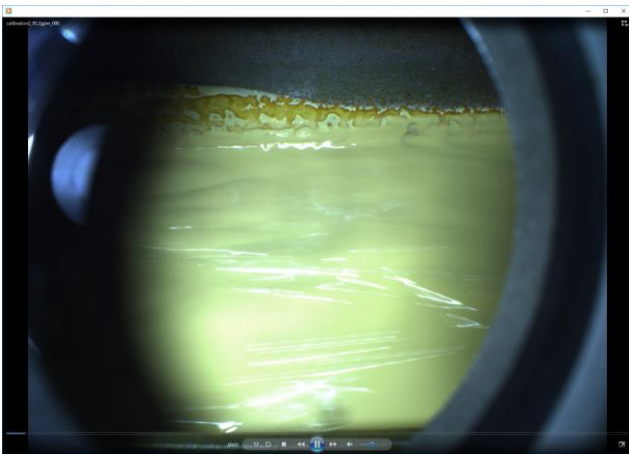
Figure 4. Image of Flow @ 95.2 GPM
